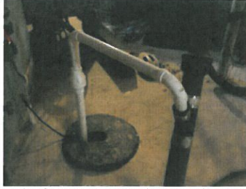
Example of sump pump hard piped to sanitary service, easily removed and redirected to surface.
