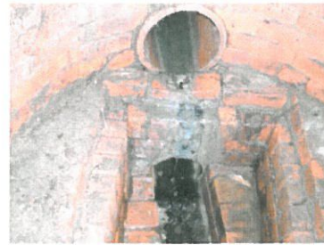
Inlet sewer and inlet drain in S75COM1515 Shows drain flowing into sewer
